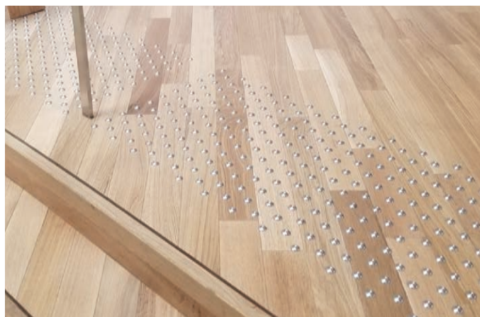
Stainless steel concentric ring domes installed on hardwood flooring.
